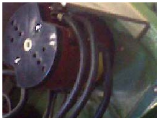
Image of the panel isolator with the unbalanced load.
